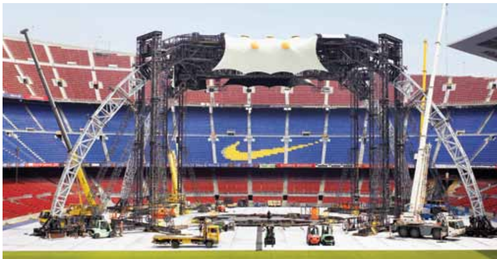
A section is added to each of the four legs after every six or seven steps
