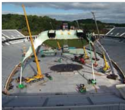
W.O. Grubb cranes lifted the steel structure into place and also constructed the surrounding light towers, sound booth, speakers and hardware
